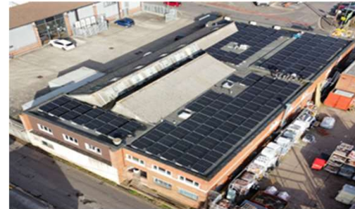
Hosiden Besson 1st phase (United Kingdom)
